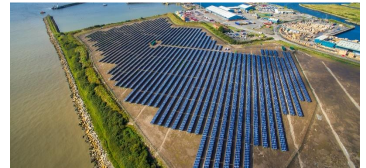
Ground Mounted Solar
